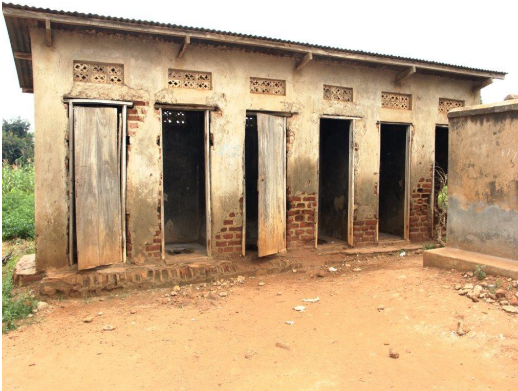
The abandoned latrine with weakened walls in Wabulungu P/S (Current pupil to latrine stance is 1:200)
